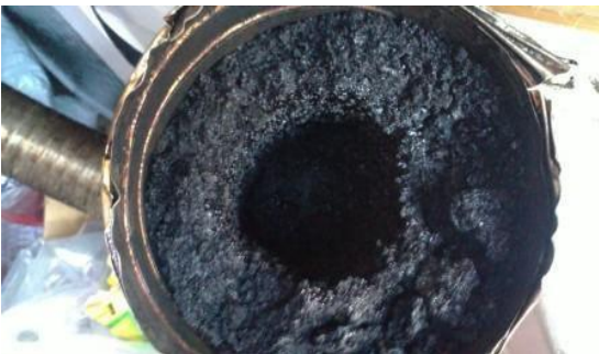
150mm chimney liner blocked with deposits
