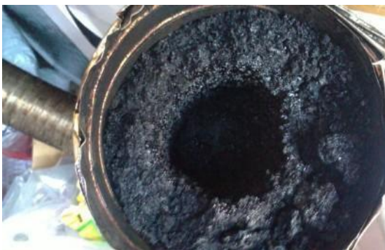
150mm chimney liner blocked with deposits
